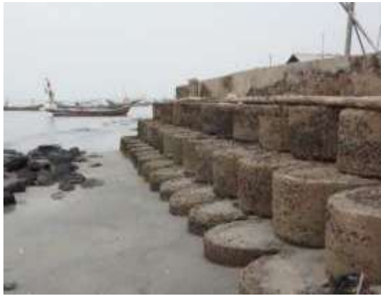
Figure 2: Sedimentation and coastal structure damages.
